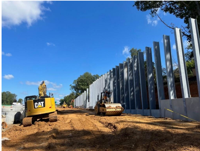
Building new noise wall along northbound I-495 between Old Dominion Drive and Georgetown Pike.
